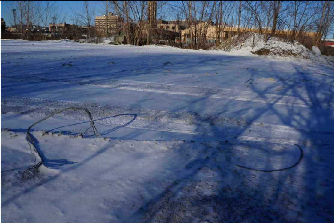
PHOTO 1: REBAR PROTRUDING FROM GROUND (TYP.)
