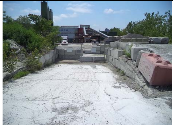
Photo 4: At the south of the platform, a fence impedes access to the platform. Fordham Road Concrete is beyond.
