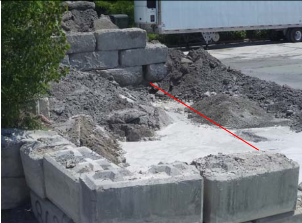
Photo 9: Accumulation of water at the southwest corner of the Site. The approximate Site boundary is shown as a red line.
